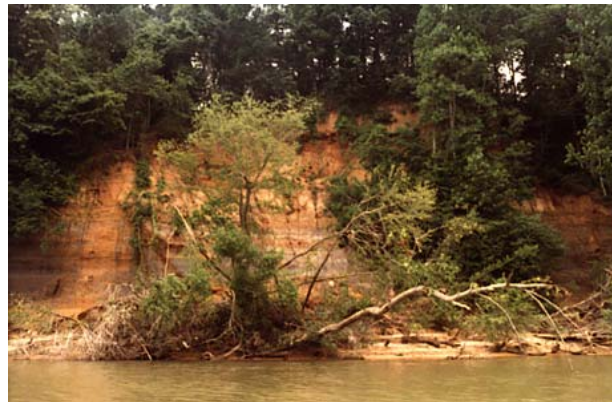
Figure 1. Example of erosion on a river bank.
