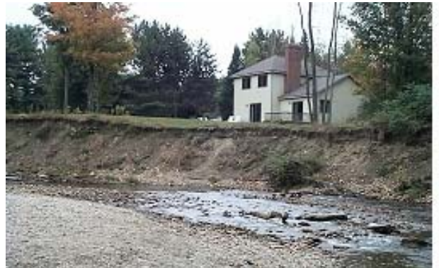
Figure 2. Additional example of erosion along a river.
