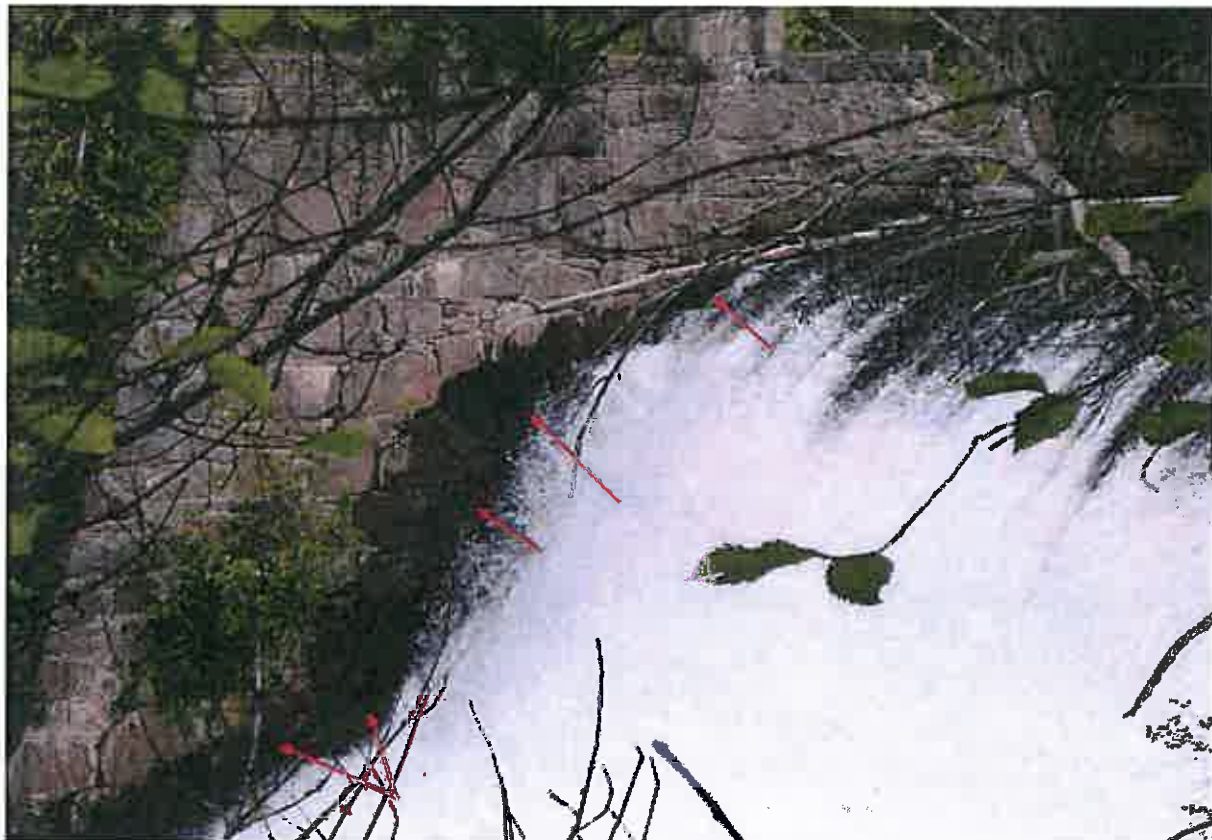
Photo 8 Dam ID# 219-1082 Rome Dam 9/14/15 Cracks, missing stone along sidewall
