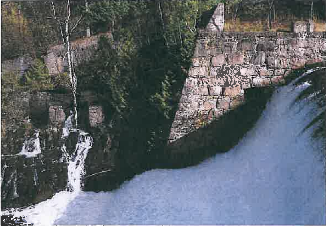
Photo 8 Dam ID# 219-1082 Rome Dam 10/22/13 Right abutment - note missing stone, mortar, leakage
