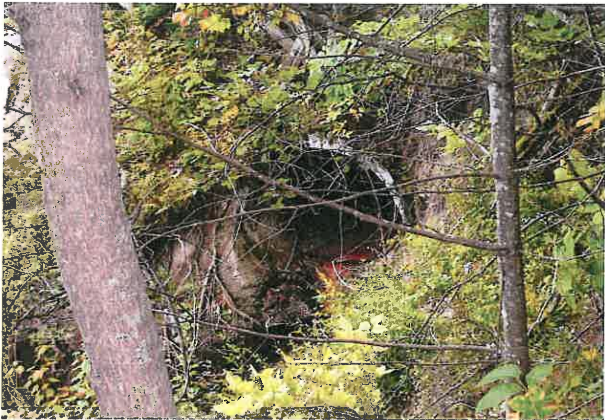
Photo 7 Dam ID# 219-1082 Rome Dam 9/14/15 Left penstock
