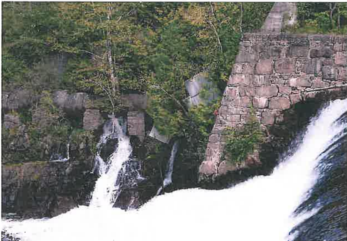
Photo 6 Dam ID# 219-1082 Rome Dam 9/14/15 Right spillway wall - note leakage through right gate, missing stone and cracks in sidewall
