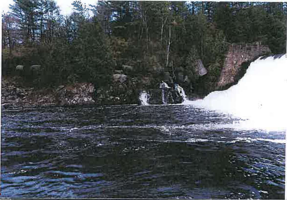
Photo 2 Dam ID# 219-1082 Rome Dam 10/22/13 Right (south) abutment/ penstock - leakage through penstock
