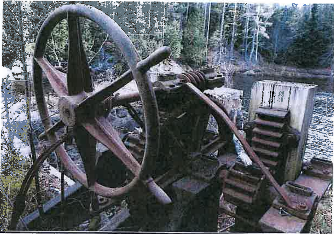
Photo 6 Dam ID# 219-1082 Rome Dam 10/22/13 Gate operator
