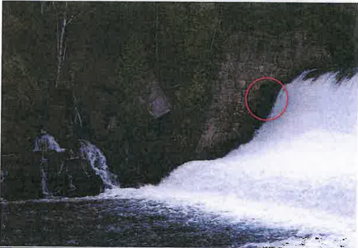
Photo 3 Dam ID# 219-1082 Rome Dam 10/22/13 Stone(s) missing in abutment, missing mortar along joints
