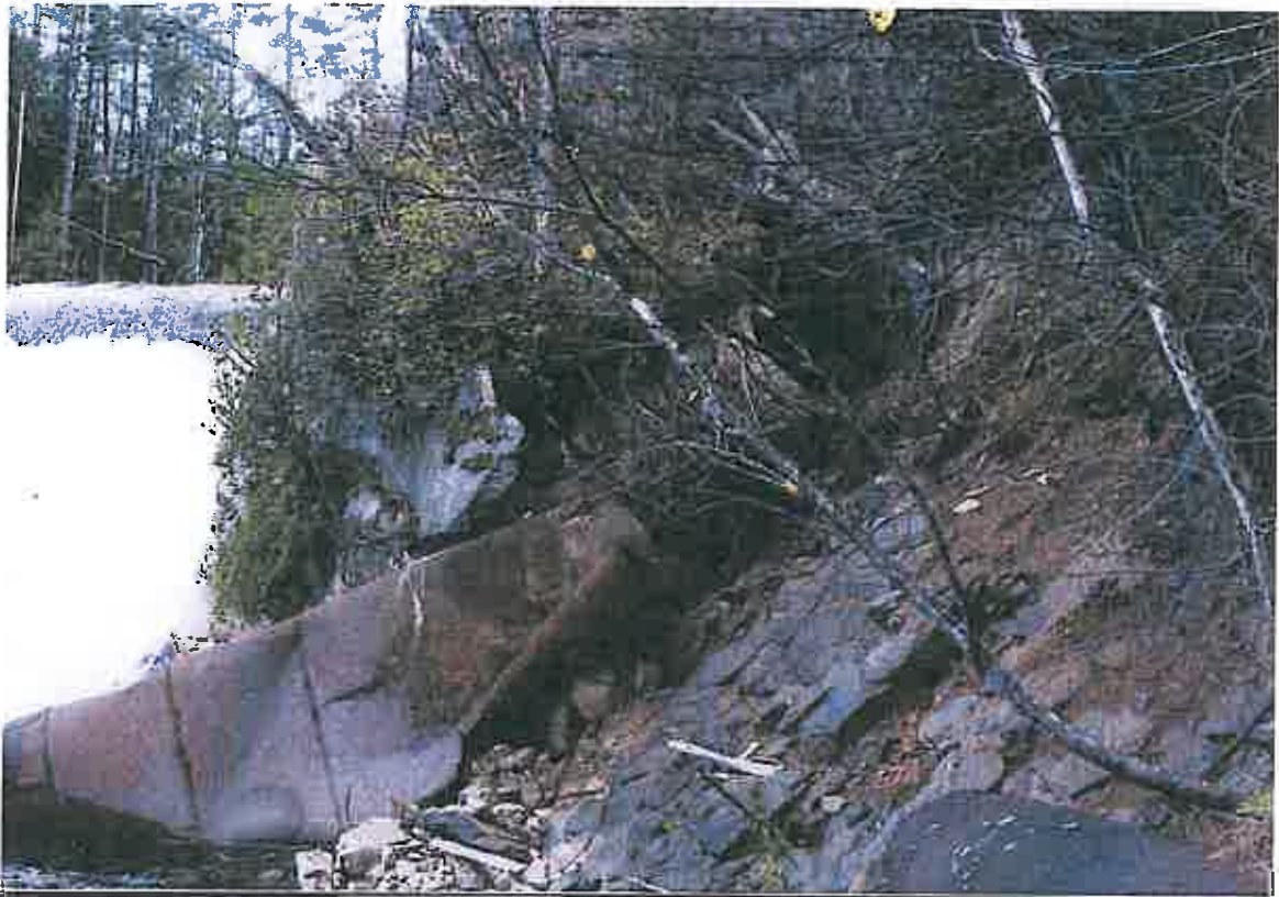
Photo 4 Dam ID# 219-1082 Rome Dam 10/22/13 Left (north) abutment downstream face - downstream concrete training wall collapsed
