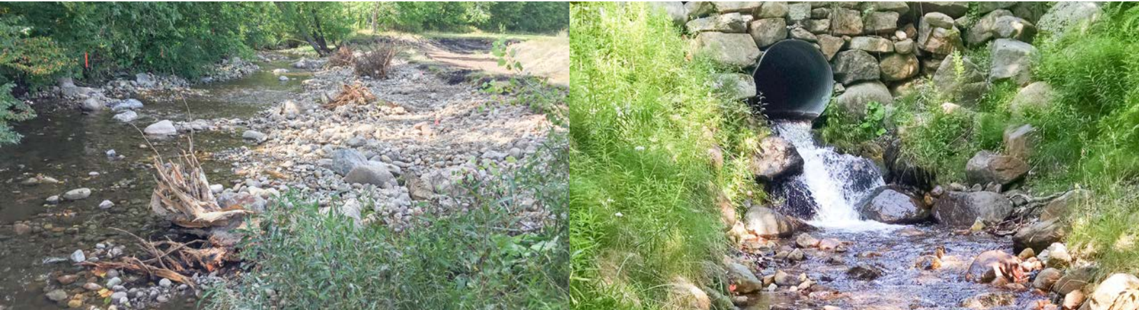
Left: Rocky Branch channel restoration. Right: Otis brook culvert before replacement, after photo in centerfold.
